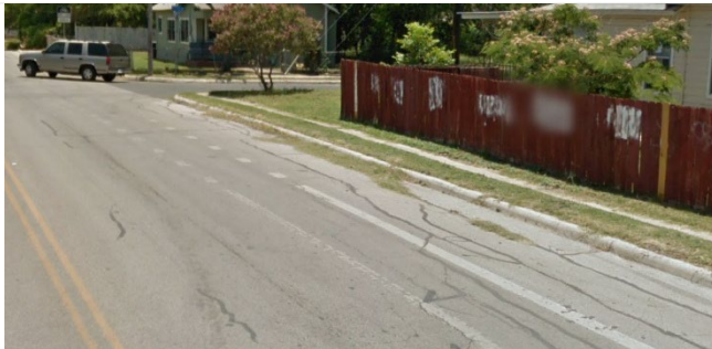
Poor asphalt conditions or landscaping overgrowth in the bikeway create uncomfortable riding conditions for people biking. Such deterioration may also encourage people to bike in the car travel lane to avoid potentially hazardous pot holes. Example on Hamilton Avenue.
