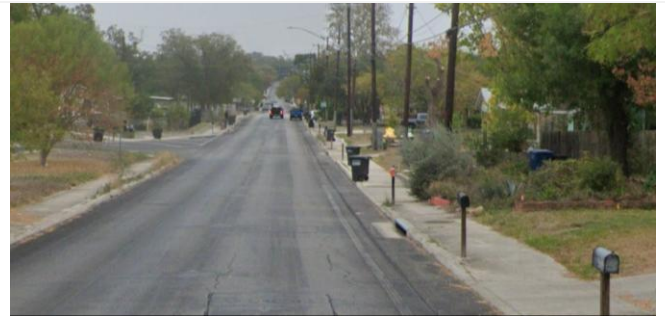
Faded bike lane striping may make it challenging for people driving and biking to differentiate between vehicle travel lanes and bike lanes. Example on Woodlawn Avenue.
