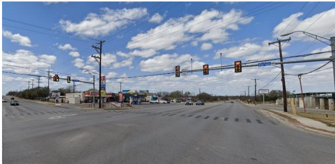
While bike lanes are present, bike lanes do not continue through the intersection nor provide any conflict striping. Example on Gillette Boulevard and Zarzamora Street
