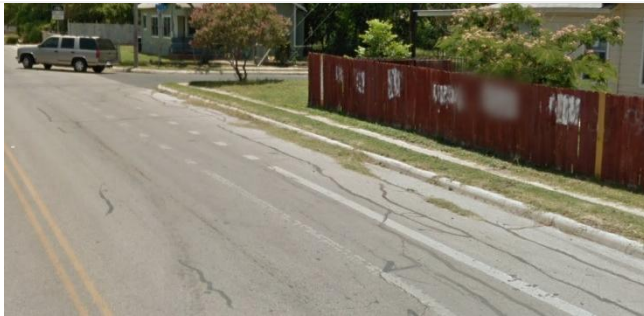
Poor asphalt conditions or landscaping overgrowth in the bikeway create uncomfortable riding conditions for people biking. Such deterioration may also encourage people to bike in the car travel lane to avoid potentially hazardous pot holes. Example on Hamilton Avenue.
